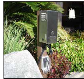
Focus Transformer Mounting
